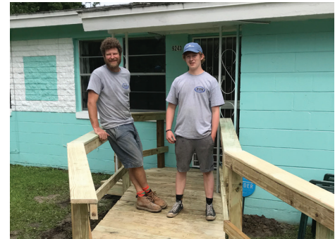
Justin Brown (left) of Builders Care is a great community partner. He helps with both ramps and home repairs.
